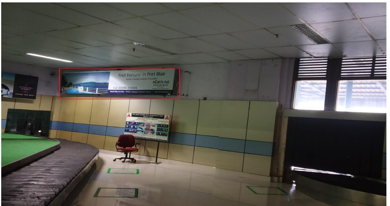
Slide No. 9 - Wall Portion in Arrival Hall Near Baggage Belt (5m x1m) (53.82 sq. ft)
