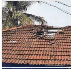
FLIGHT PATH: Tiles go off the roof of a house near Kochi int'l airport
