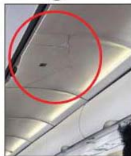
SAFETY CRACKS: AI flight 2379
