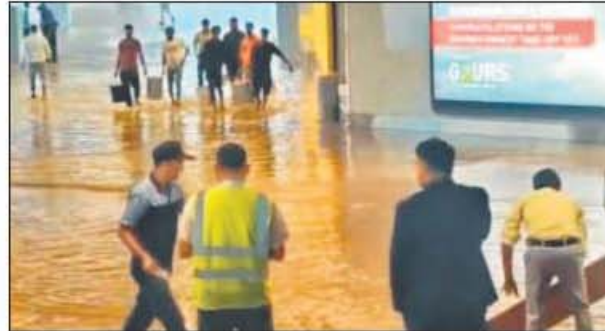
Rainwater entered the passage connecting the arrivals area and the parking bay. SOURCED
